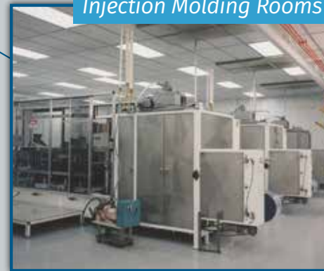
Injection Molding Rooms
