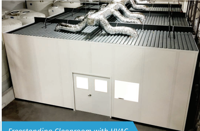
Freestanding Cleanroom with HVAC
